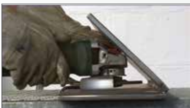
Typical problem...Grinder doesn't reach
