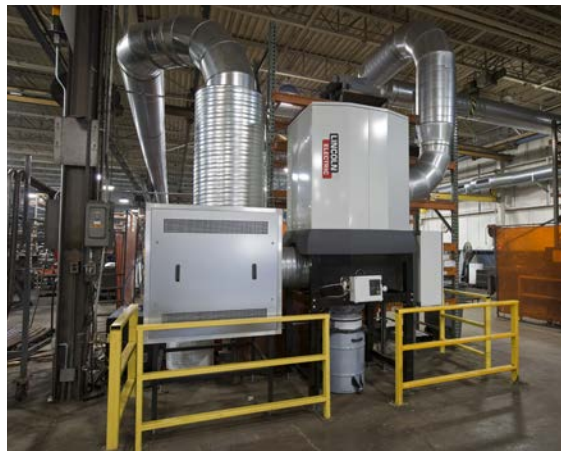
Push/Pull System installed at Elgin Sweeper Company
